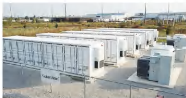
Brazil Power auxiliary service energy storage project
