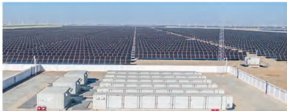
10MW 20 Sets Distributed ESS Cabinet Kenya Power auxiliary service energy storage project
