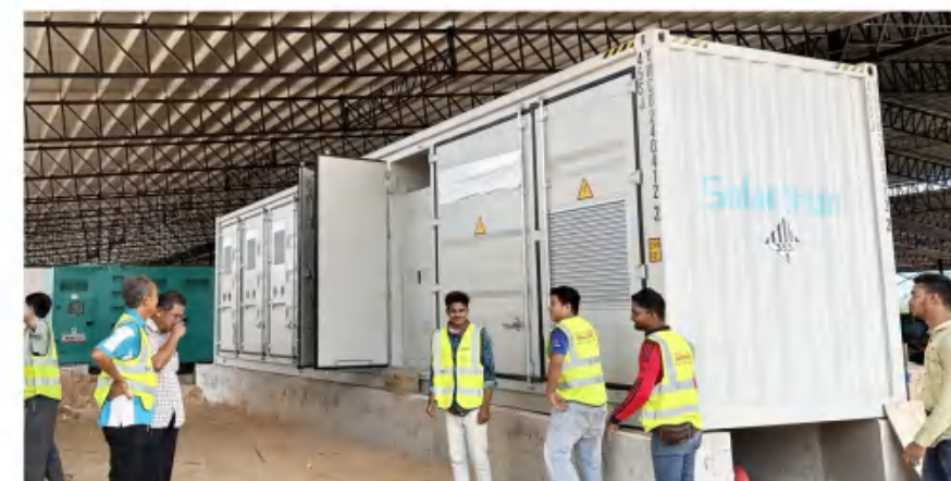
Malaysia Power auxiliary service energy storage project
