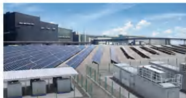
Brazil Power auxiliary service energy storage project
