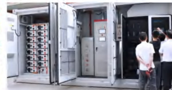
Brazil Power auxiliary service energy storage project
