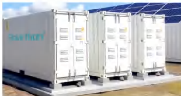
10MW DISTRIBUTED CABINET
