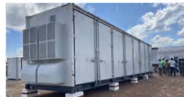
Brazil Power auxiliary service energy storage project
