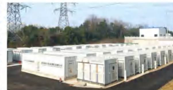
Brazil Power auxiliary service energy storage project
