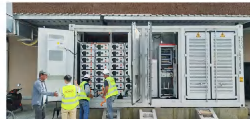
Malaysia Power auxiliary service energy storage project
