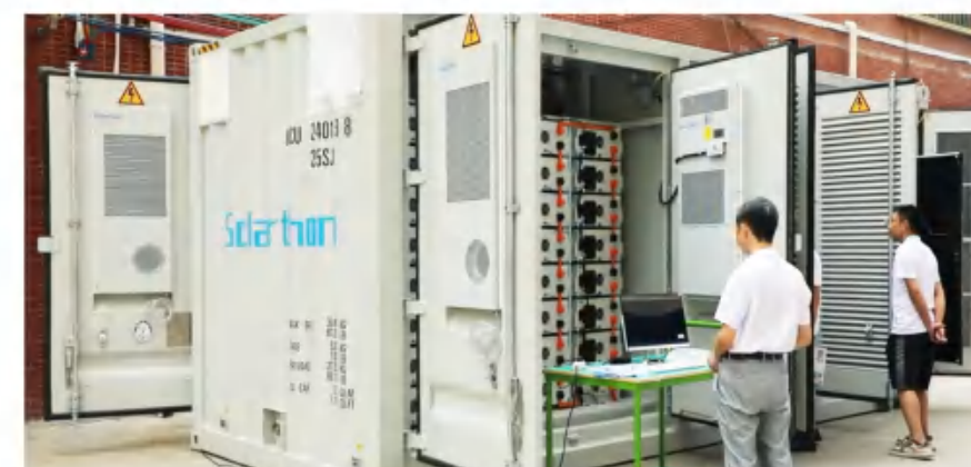
Malaysia Power auxiliary service energy storage project
