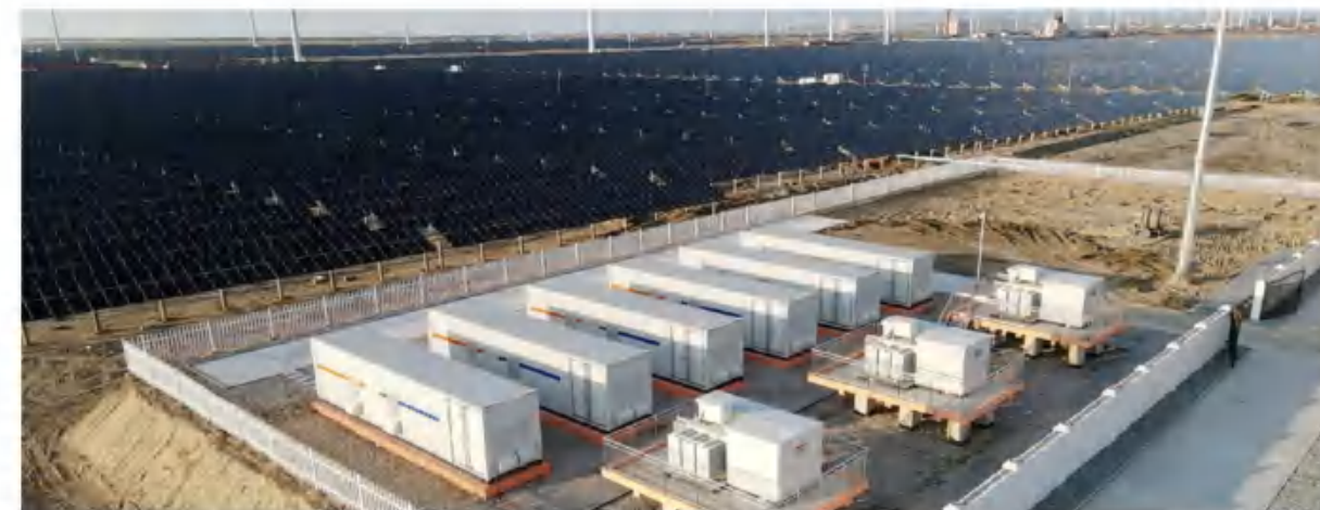
100MW/200MWh Kenya Power auxiliary service energy storage project
