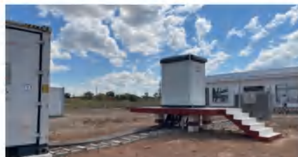
10MW DISTRIBUTED CABINET
